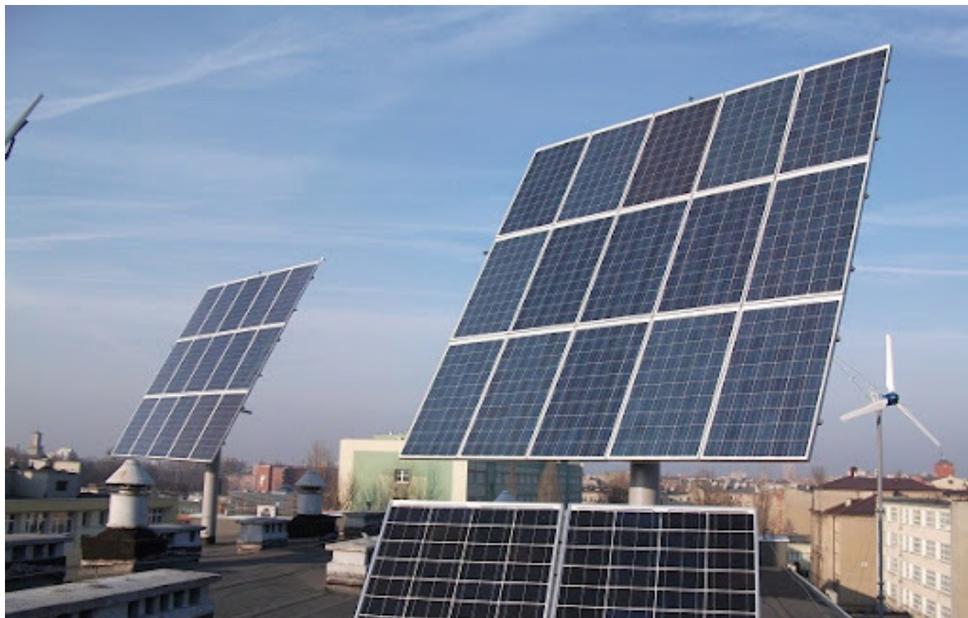
Photovoltaic installations on the roof of the TUL Faculty of Electrical, Electronic, Computer and Control Engineering building Source: TUL resources
